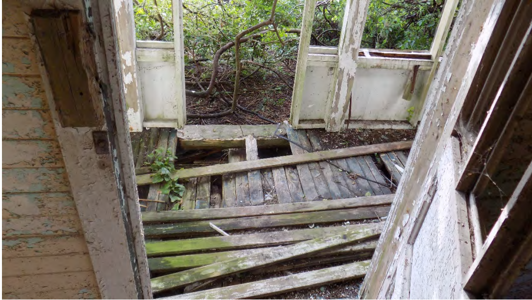
Figure 24. Caretaker's Cottage front porch, viewing east. The porch is in severe disrepair and unsafe to walk upon.
