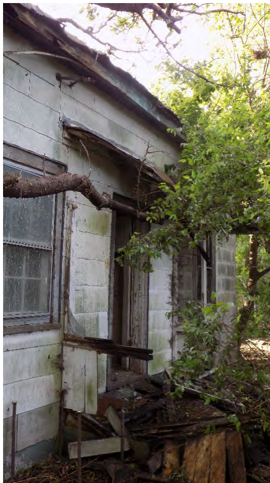
Figure 25. Caretaker's Cottage back porch, facing south-southeast. The overhang has almost completely collapsed. The threshold is covered in debris and rotting wood.
