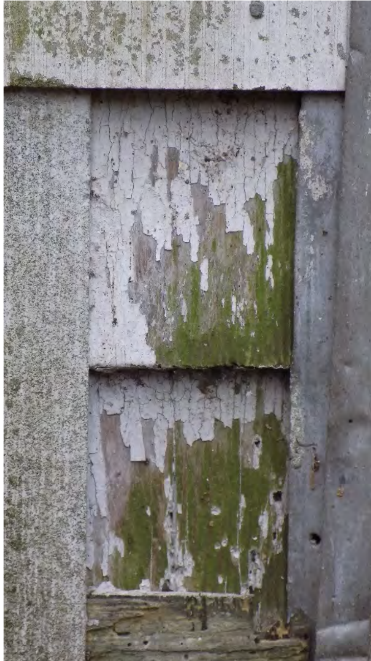
Figure 22. The wooden shingles underlying the asbestos shingles can be seen in portions along the building's northern elevation.
