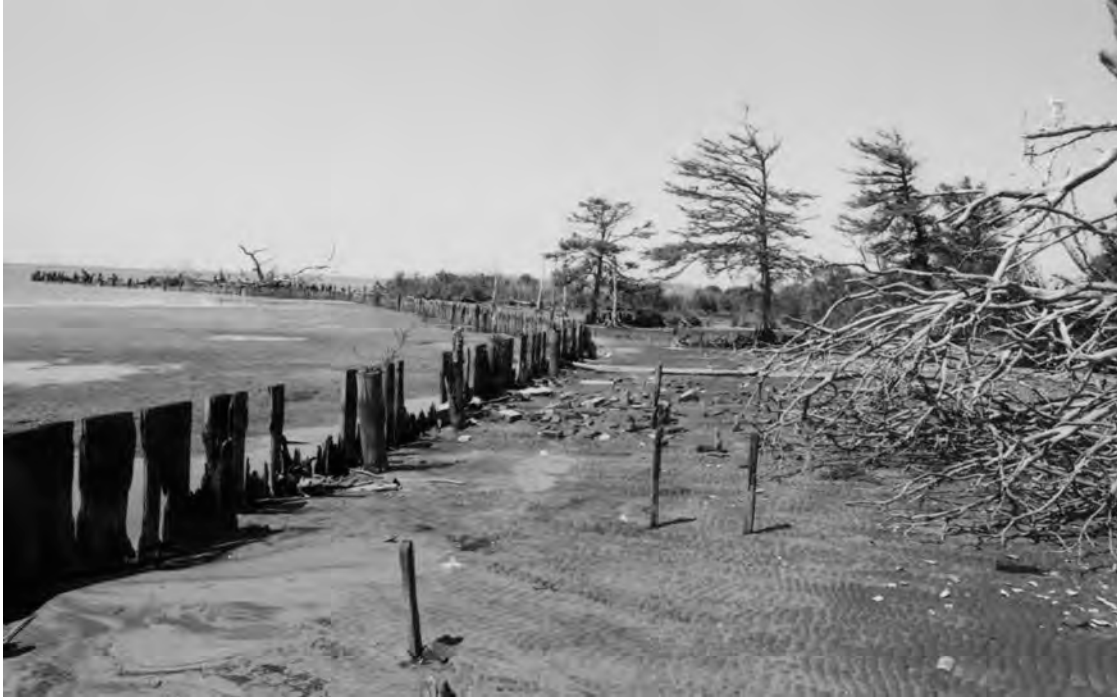
Figure 5. Failed wood bulkhead, west side of Monkey Island [Source: Kanaski 2001].
