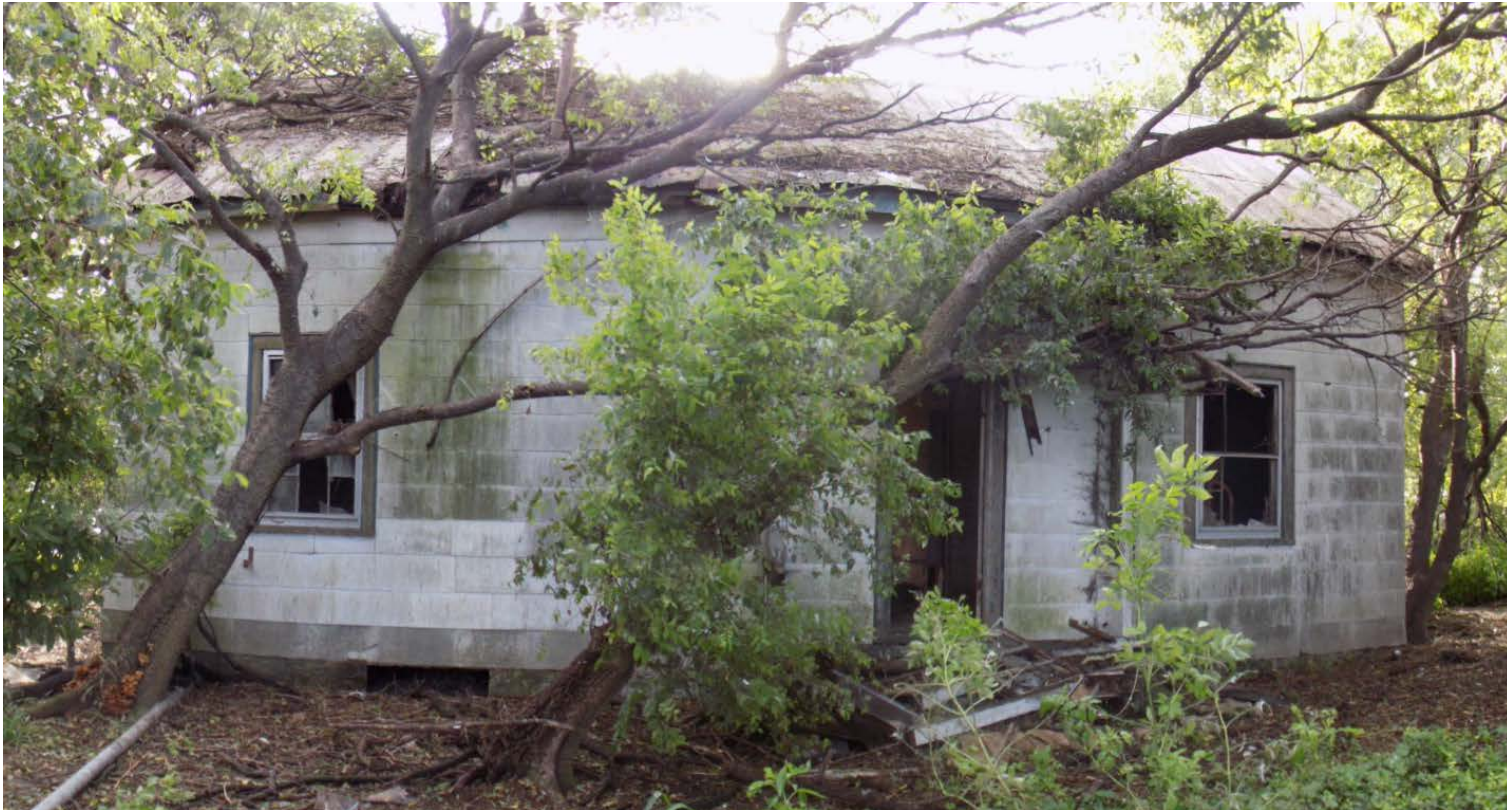
Figure 19. Caretaker's Cottage, western elevation. Many windows have been broken and the back porch overhang has collapsed. Fallen trees and limbs have damaged portions of the roof.
